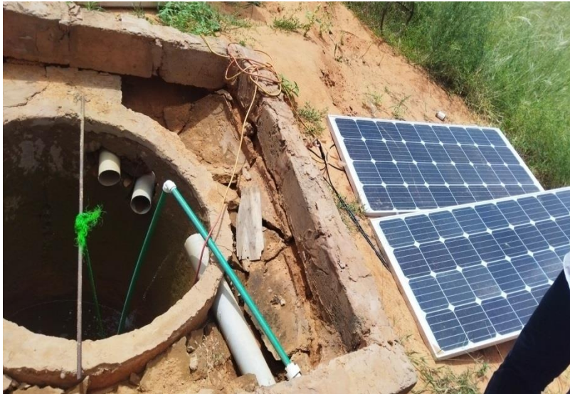
Water recovery system 1
