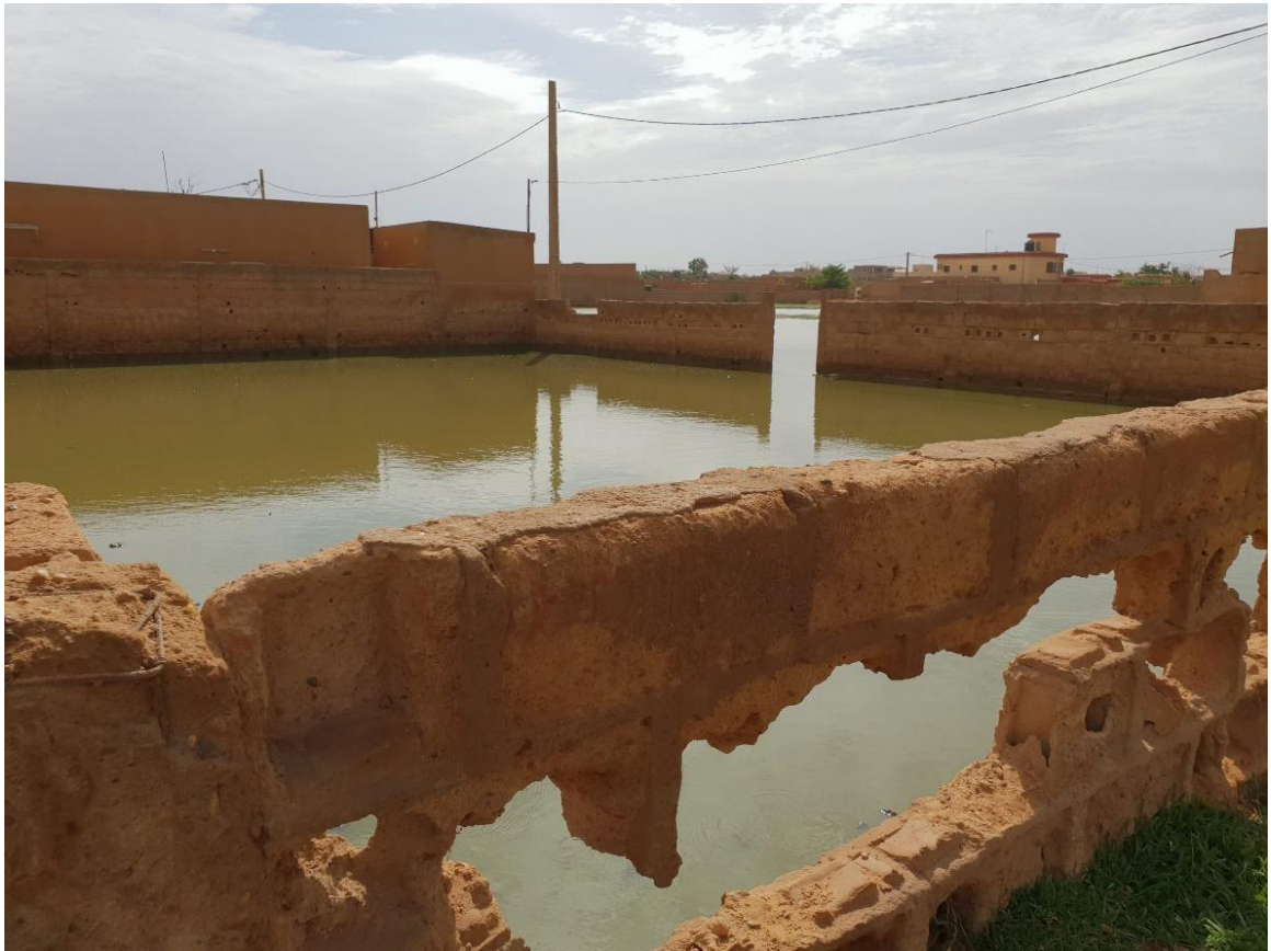
Plate V: A house flooded by the rising water table in the Sonuci district (Niamey, July 3, 2020) source: https://www.studiokalangou.org/13062-niamey-inondations-quartiers-sonuci
