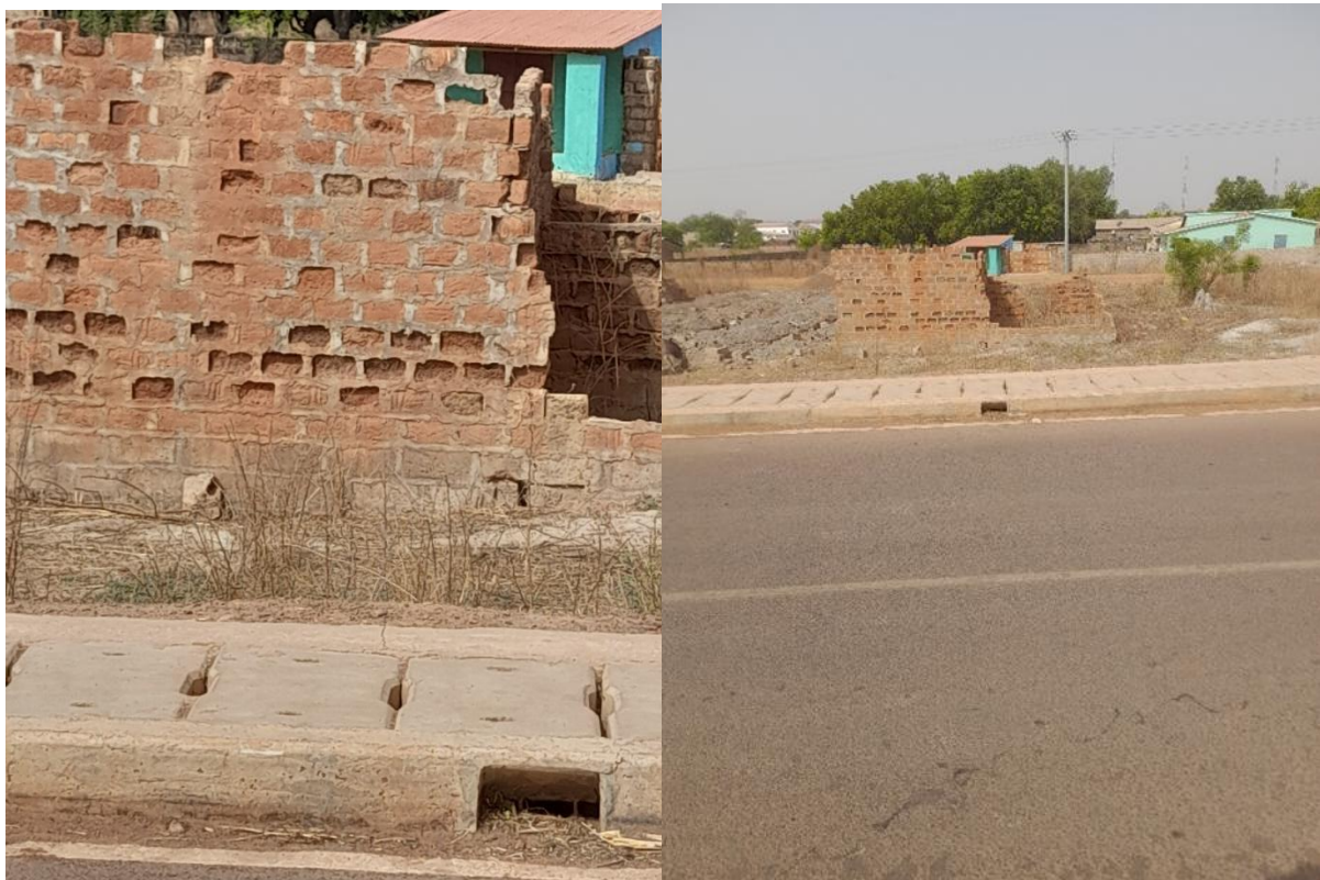
Figure 8: A sample of a mod house built with a strong foundation of cement brisk but was deroofed by a wind storm in Kaba-Kamba, URR South, (author's own, June 2023)
