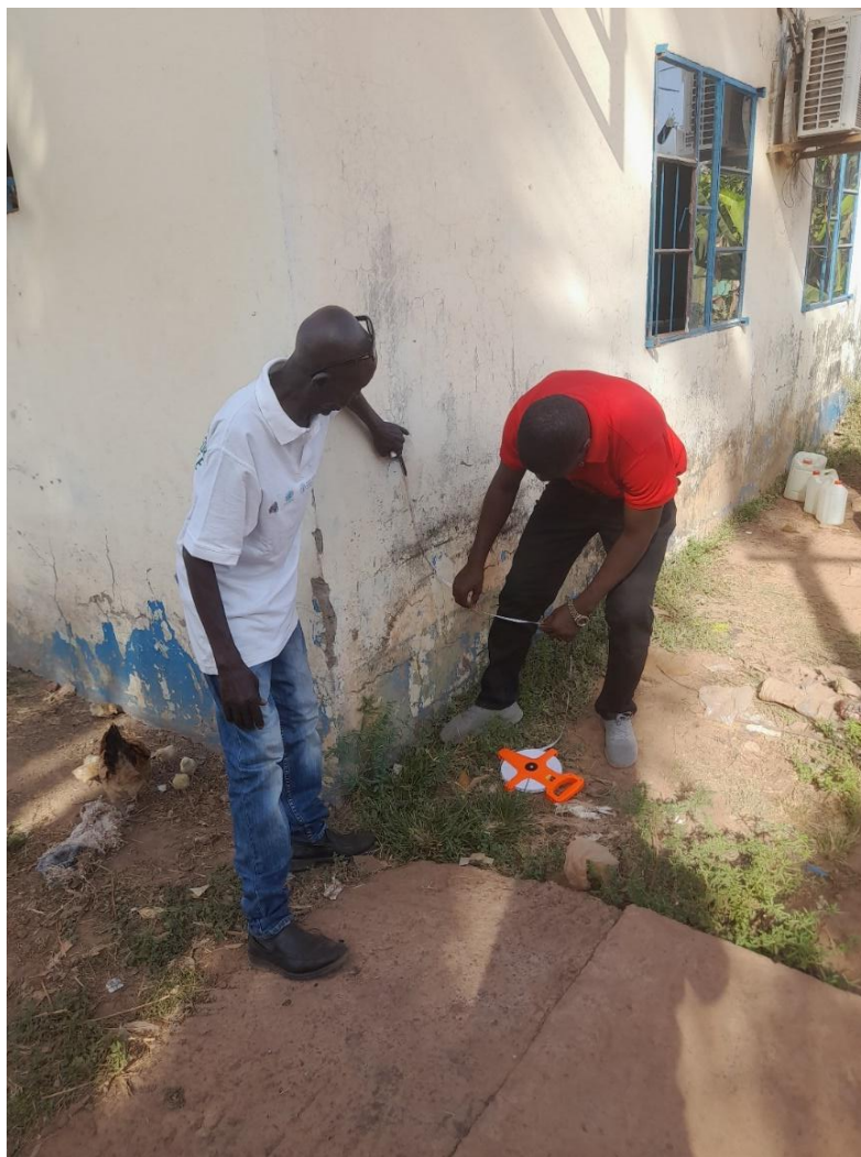
Figure 6: A man in Kuntaur Wharf Town (CRR North) indicated water levels on wall bricks during flooding in 2022.
