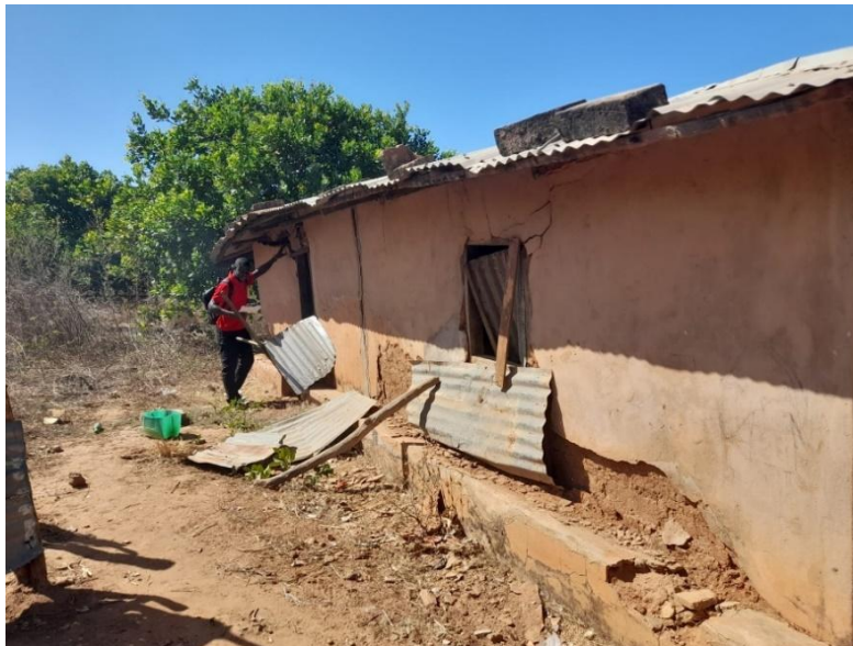
Figure 10: A sample of that collapse and the owner can afford to rebuild and use a temporary corrugated sheet in Faraba-Banta WCR (author's own, November 2023)
