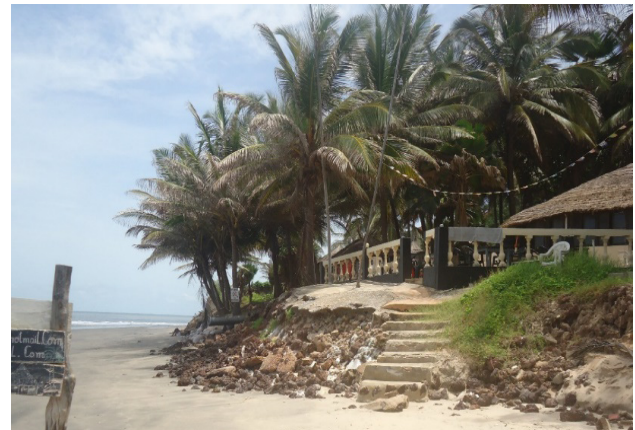
Figure 8. Some Structures at Risk of Coastal Erosion. Source: Author, 2017
