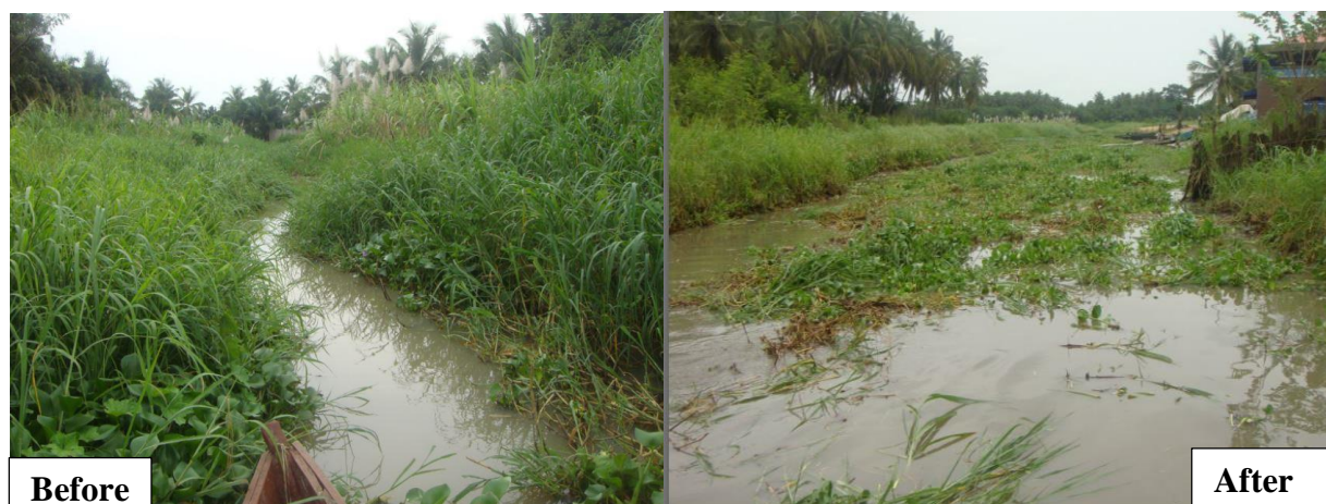
Dredging of a stream at Agbanakin to allow smooth flow of water
