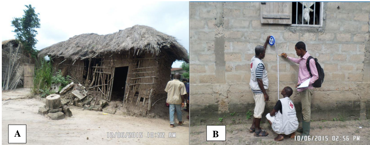
(A), An abandoned house at Azime Dossou due to flooding. (B), Measuring floodwater height at Agbanakin
