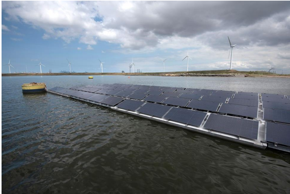
Figure 3.4-2: Floating PV system on a water body in Netherlands
